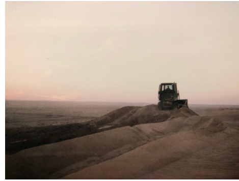
Camp Rhino Dozer Operations: Excavating borrow pits and making fighting position improvements, 2001. Photo taken by IT3 Martin Reiger.
