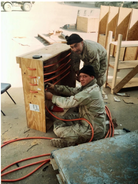
Rhino Camp Improvements: CE1 Victor Cabrera and CE3 Stuart Dahl making expedient "distribution panel" for transitioning power between generators. Photo taken by IT3 Martin Reiger.
