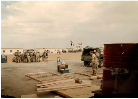
Camp Rhino: Seabees constructing 4-Hole Burnouts. Note New York state flag flying under U.S. flag in background, 2001. Photo taken by IT3 Martin Reiger.
