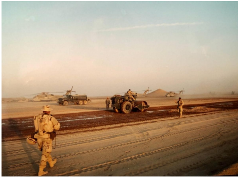
Rhino Airfield Repairs: Roller and Water Truck Ops, 2001. Photo taken by IT3 Martin Reiger.
